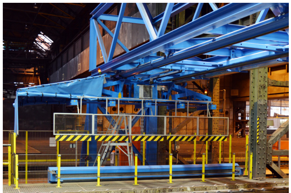
Figure 7. The measuring beam – with the five sensor units – in the parking position. Installed below is the calibration block in hard stone (Picture: Salzgitter Mannesmann Grobblech)
