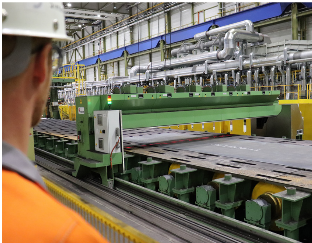
With almost 30 meters in length, the flatness measuring system installed downstream the new RM 5 levelling machine is the largest measuring system ever built by nokra (Picture: Ilseburger Grobblech GmbH)
