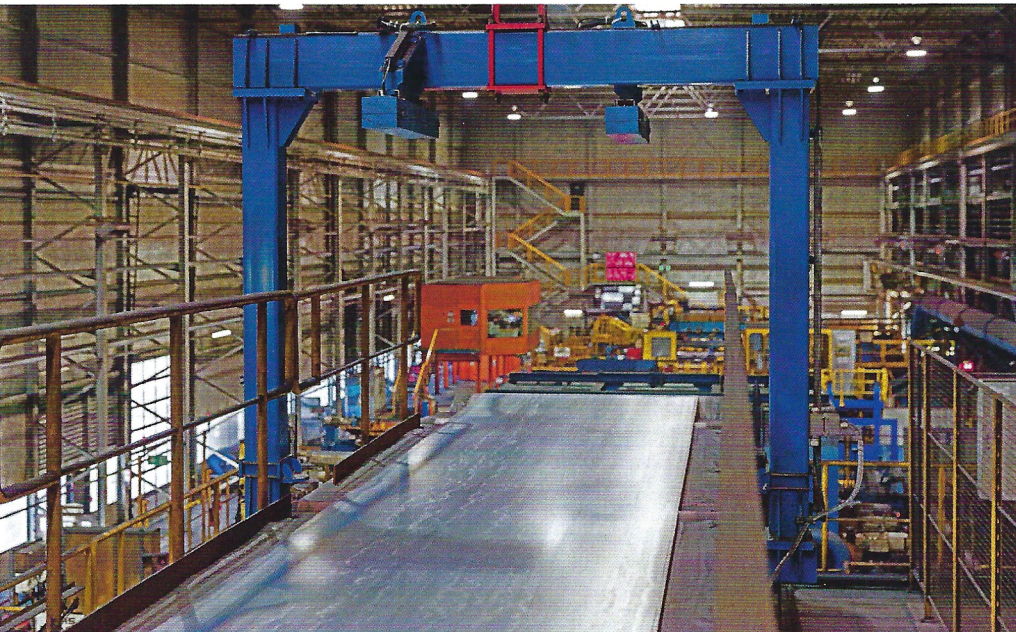
The entry gauge is arranged between the bridle rolls and the entry of the pickling section (Picture: Salzgitter Flachstahl)
